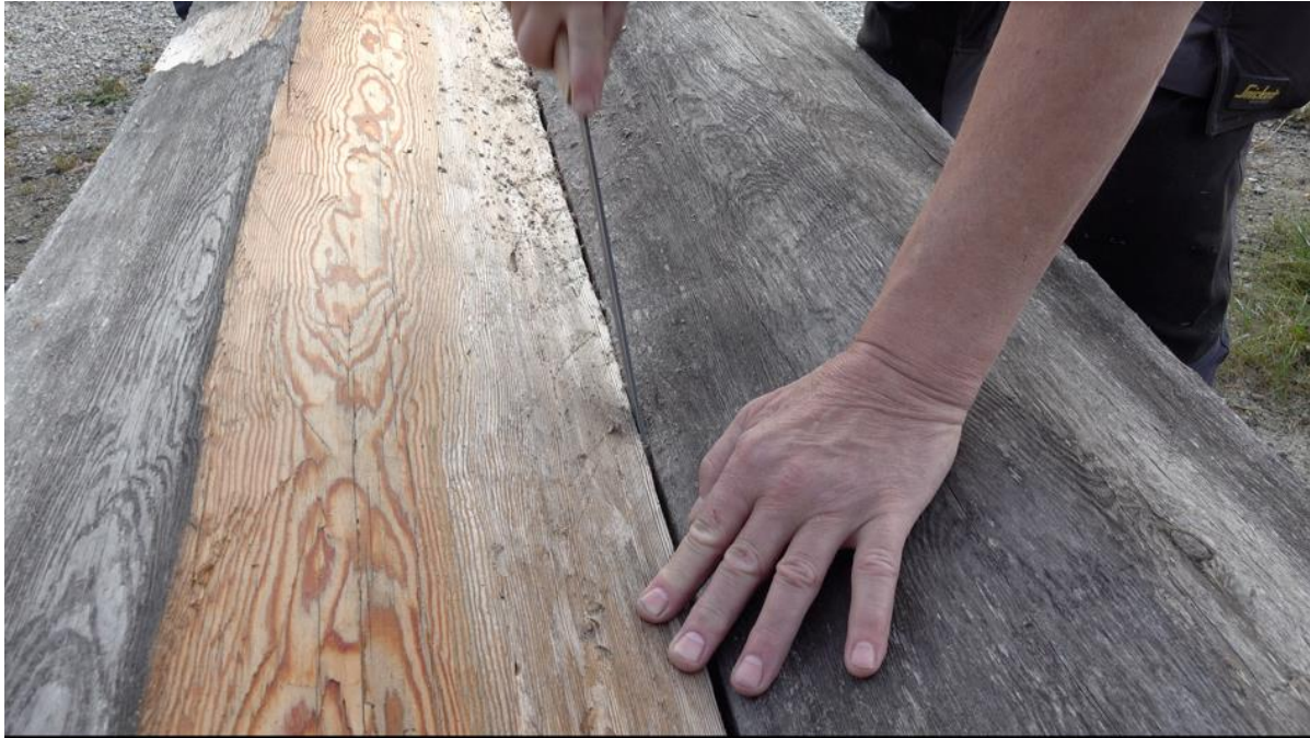
FIGURE 11. Testing of a hypothesis of using the saw, to joining the wall staves with a tight seam.
