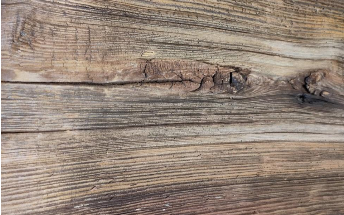
FIGURE 7. Checks in the pith area of the tree, on an uncoated board of Pine, from a board-on-board cladding of the South façade of a log house in Örnäs, Skåne, Sweden, from 1865 to 1880. Erosion of the early wood is also observable, while the hard latewood remains, its fibres standing perpendicular to the weathered surface (Almevik, 2012, p. 115). Erosion is a slow process caused primarily by the photodegradation of lignin (by ultraviolet and visible light) and increased by rain and water (Sell et al., 1986, p. 57).
