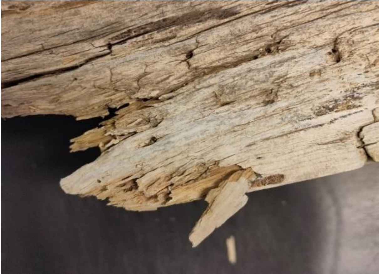
FIGURE 4. A sample from the South façade of a barn built with log walls in Västra Götalands, Sweden, and clad with standing boards of Alder. It shows rot in the part that used to be close to the ground. There is no trace of paint and it is likely that it has always been uncoated. Most of the boards are still fixed on the walls today, but they present a large number of insect holes (see Figure 6), especially on the north side, and some rot on the lowest parts of the walls.
