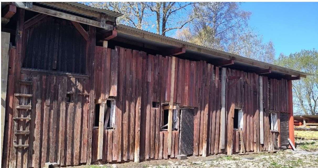
FIGURE 3. The stable of Kvibergsnäs, Sweden, was built in the 1780s and its East façade tells many stories. Figure 5 shows an exhibited sample from a panel board belonging to this façade.
