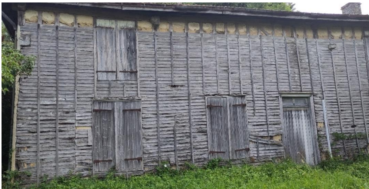
FIGURE 1. The South-East façade of a house built with timber-framing and wattle and daub filling in Outines, Champagne, France. Tavillons are thin slices of wood cladding the façade, traditionally the most exposed to rain or, like here, facing the main street. They overlap in a horizontal pattern, held in place by vertical wood battens, and often stop a good distance from the roof where they are not needed. They prevent the porous wattle and daub filling from constantly swelling and retracting, making the construction less and less air- and watertight.
